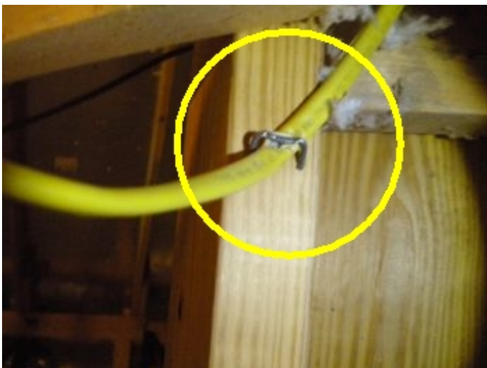
Romex wire sheathing torn – Recommend repair by qualified professional
