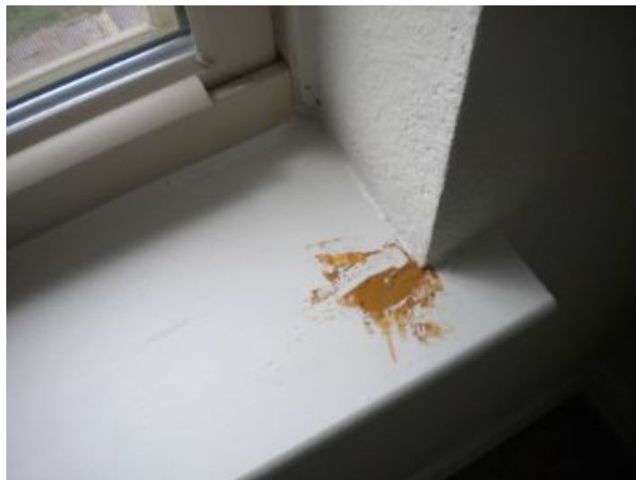
Trim under window has been patched
