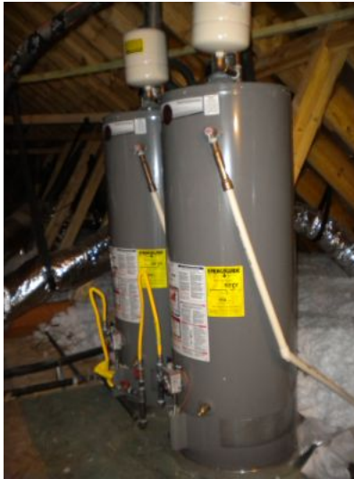
Dual 50 gallon gas water heaters located in attic
