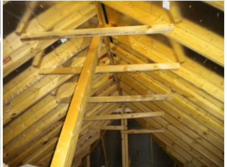
The attic structure was observed to be conventionally framed with rafters, purlins and collar ties
