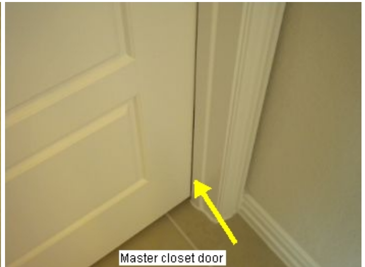
One or more doors were observed to have gap at jamb.
