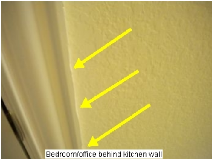
One or more doors casing trim showed evidence of damage
