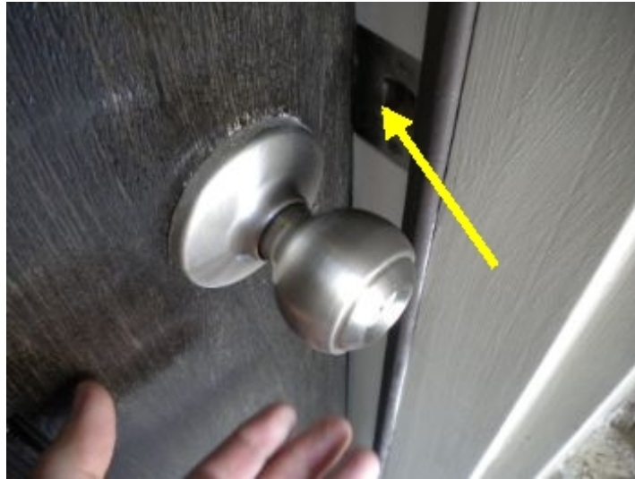
Front door handle hard to turn when fully closed and latched - Recommend adjusting strike plate to make handle easier to turn.
