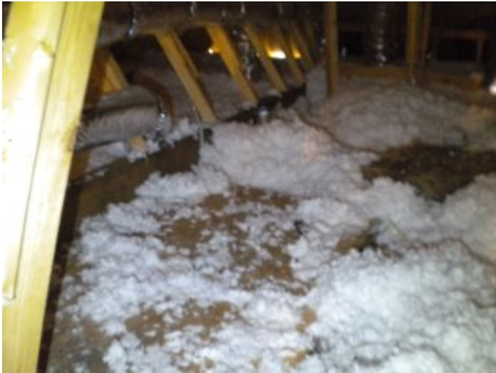
Suggest checking insulation depth under this plywood in attic.
