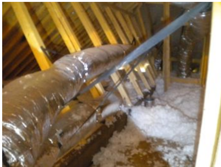
Duct work in attic
